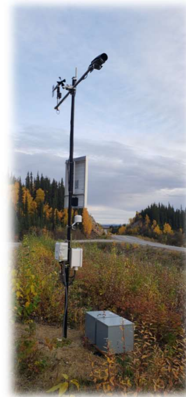
Mini-RWIS Station, Alaska Highway MP 1285
